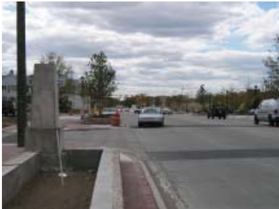
Looking west along Auburn Road at Juniper Avenue during construction of new streetscape
