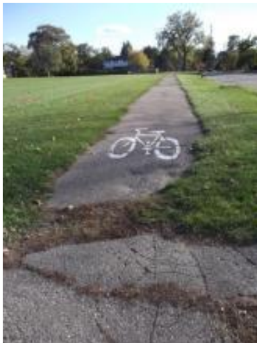
Poorly maintained landscape reduces the usability of a non-motorized path.
