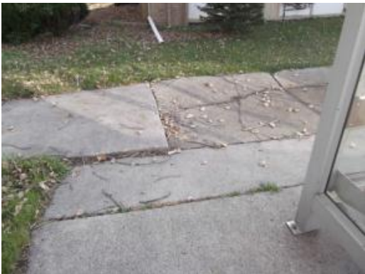
Many existing concrete pads are in need of repair.
