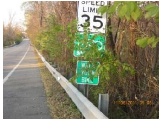
While not directly affecting the path, overgrown landscape can interfere with usage by reducing wayfinding sign visibility.
