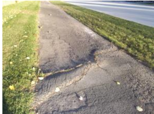
Settling and tree routes often interfere with the safety of a non-motorized path.
