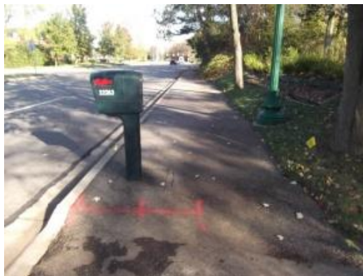
Permanent objects sometime interfere with safe pathway use.
