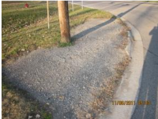
This pedestrian pad is constructed of inadequate materials, creating safety and maintenance issues.
