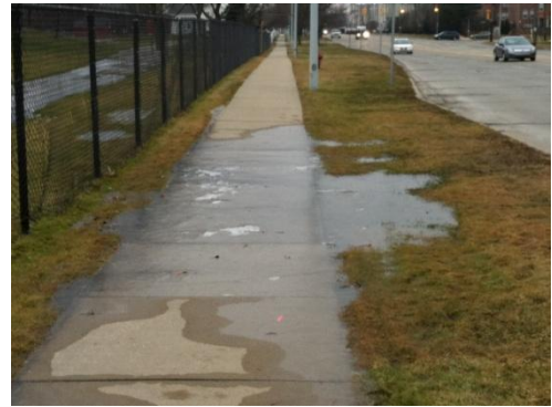
Lack of drainage results in wet, slippery pathways that are often not passable.
