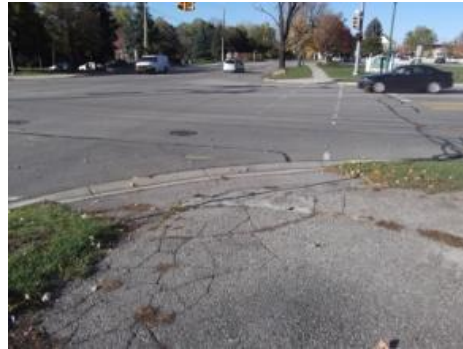
Painted crosswalks are worn and nearly invisible.
